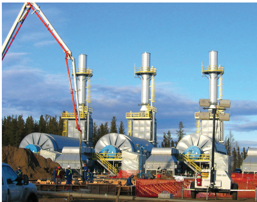
Construction workers busy at a Vista Projects SAGD project in the Alberta oil sands. Photo courtesy Vista Projects Ltd.
